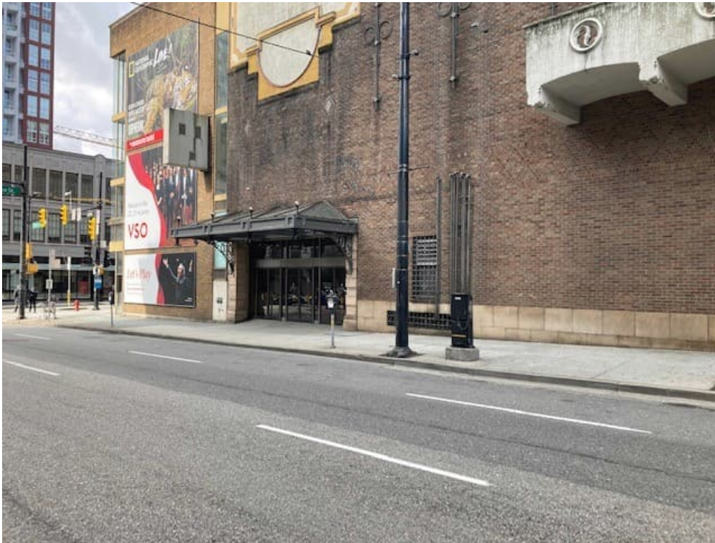
Street Bus Parking With Shore Power Box
